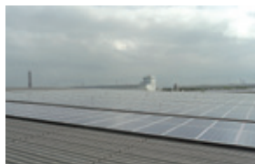
Solar power generation (JSAI: India)
