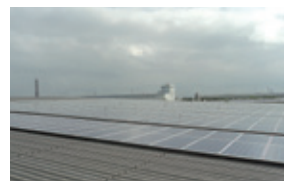
Solar power generation (JSAI: India)
