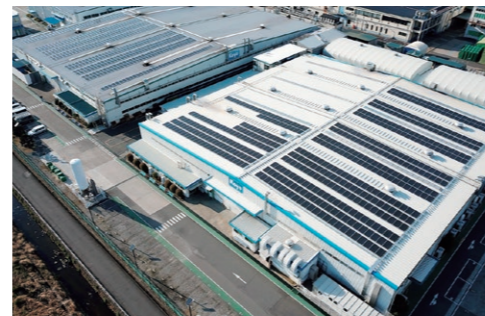
Solar power generation at Koyo Machine Industries Co., Ltd.'s Yuzaki Plant
