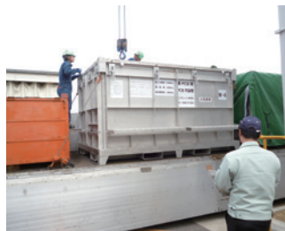
PCB ballast treatment status (Kariya Plant)
