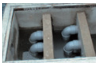
Oil-water separation device
