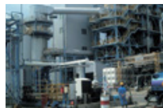
On-site check of incineration facility (July 2005)
