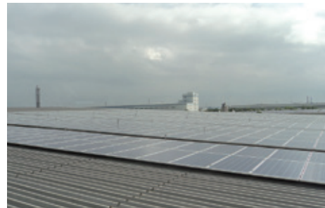
Solar power generation (JSAI: India)
