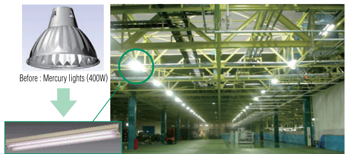
High-efficiency fluorescent lights (Four Hf 32W bulbs) [Kariya Plant / Higashi-Kariya Plant / Hanazono Plant]
