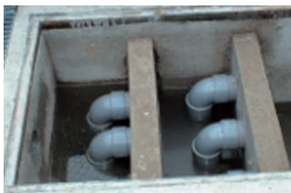
Oil-water separation device
