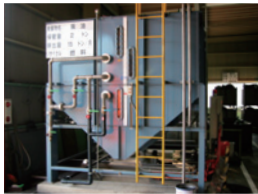
Oil-water separating tank
