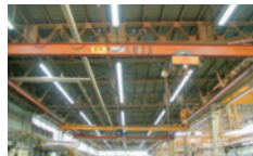
Inverter-controlled fluorescent lights
