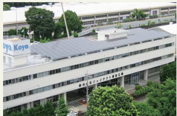
Solar power generation (Tokyo plant)
