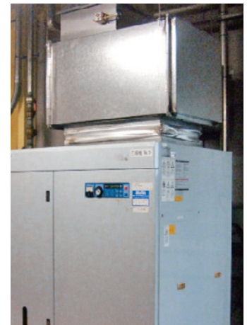
Installed a duct on the compressor (New south plant on our Tadomisaki site)
