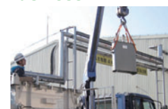
Status of PCB device treatment (Tokyo plant)
