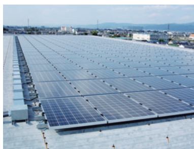
Solar power generation (Nara plant)
