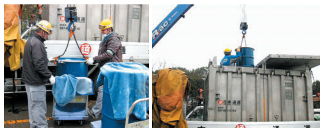
PCB ballast treatment status (Tokushima Plant)
