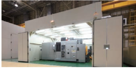
Fig. 5 Large-sized environmental test room
