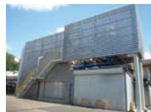
Cogeneration system at Kokubu Plant
