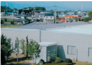
Solar power generation (Tokushima plant)
