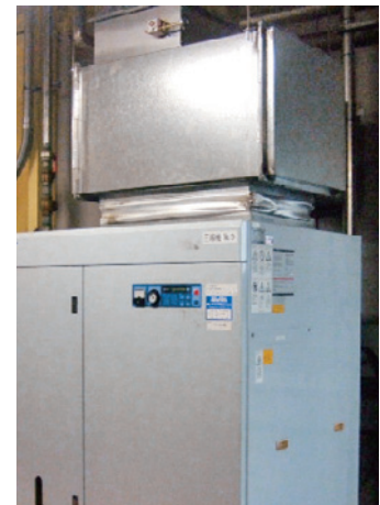
Installed a duct on the compressor (New south plant on our Tadomisaki site)
