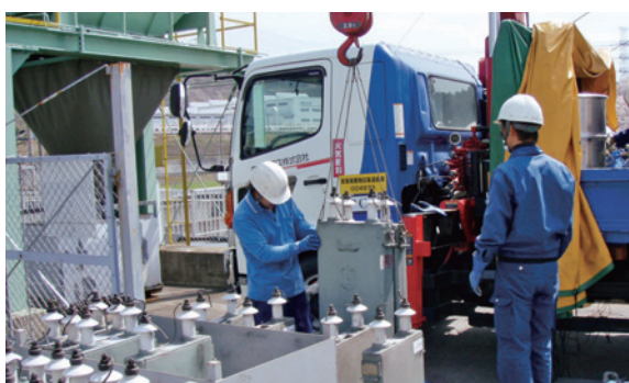
Status of PCB device treatment (Okazaki plant)
