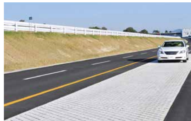
亀甲路 Cracked Surface Course
